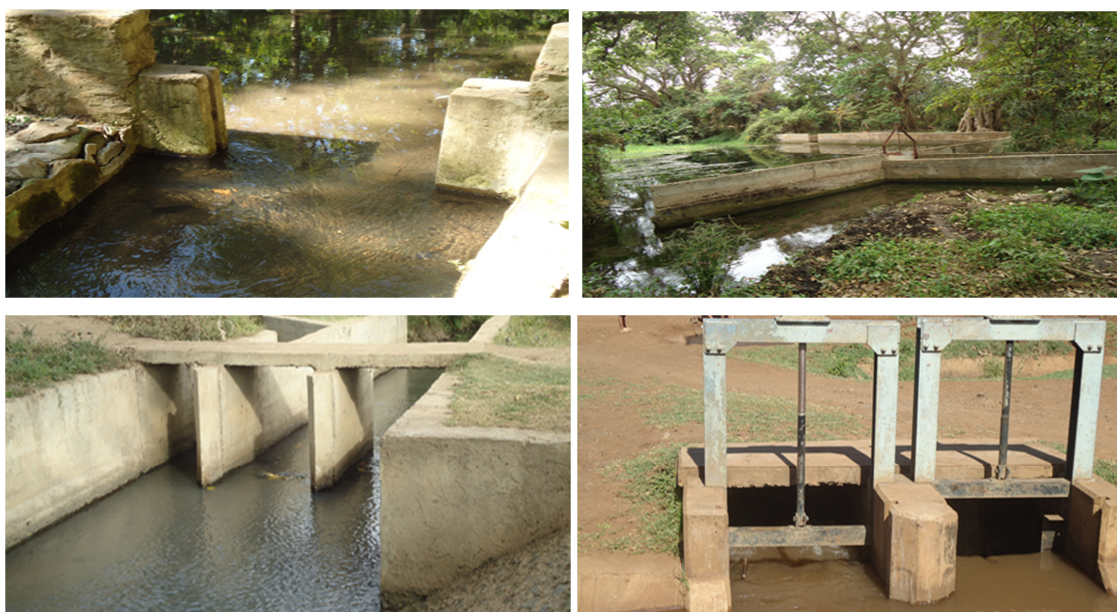
Figure 6: Water intakes for irrigation canals along the PRB, Tanzania
