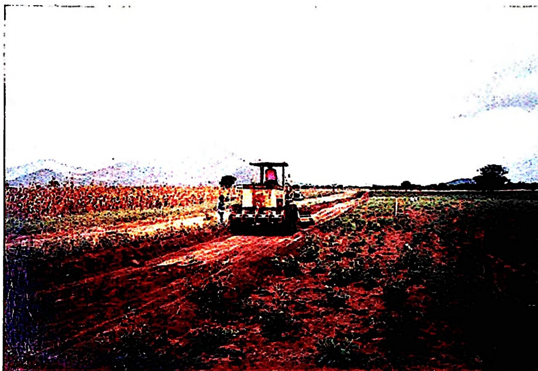
Figure 5.8. Construction of a grassed waterway to drain water from the contours on field 15.
